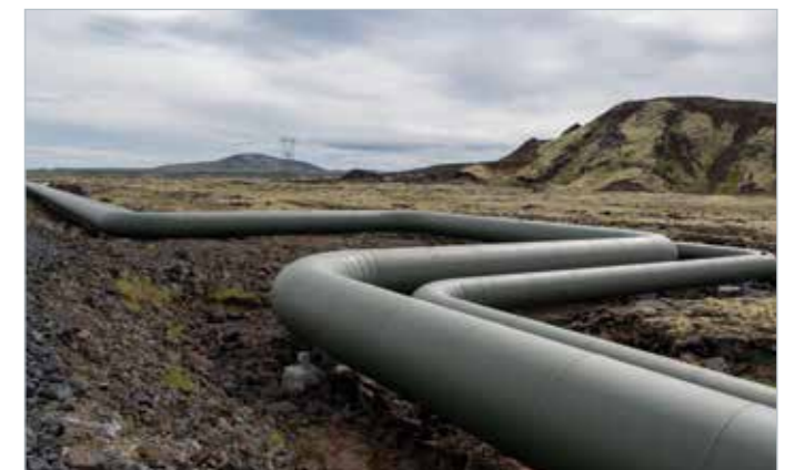
District heating supply
