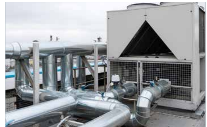
Building cooling systems
