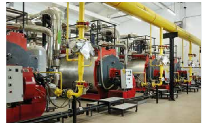
Large-scale heating systems
